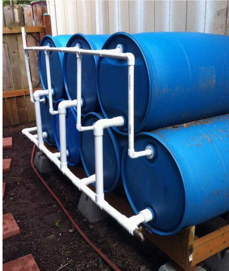
Fig 84: The rainwater collection system below is at Humble Parquito in Chicago. Their sophisticated system provides up to 80% of their water year round.
